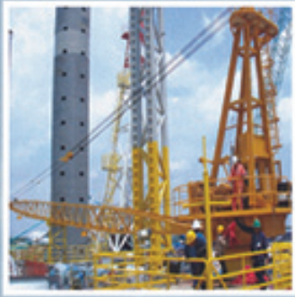
Cendor field Development MOPU Conversion 40-man Living Quarters, Terengganu Malaysia.
